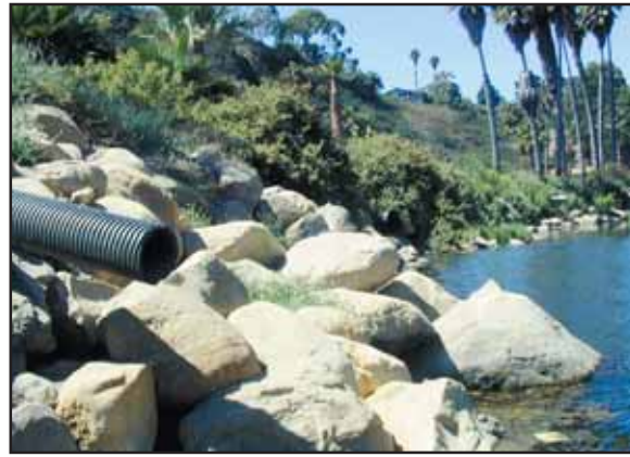
This storm drain empties water from the parking lot at Arroyo Burro Beach right into the creek.
